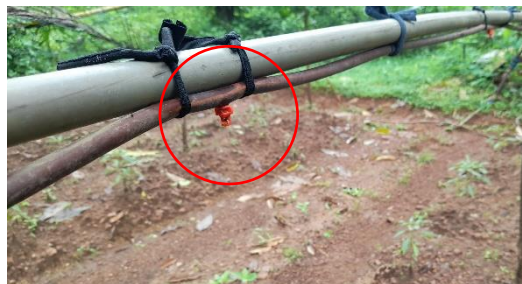
Figure 6: Water distribution pipe network & spray nozzle.
