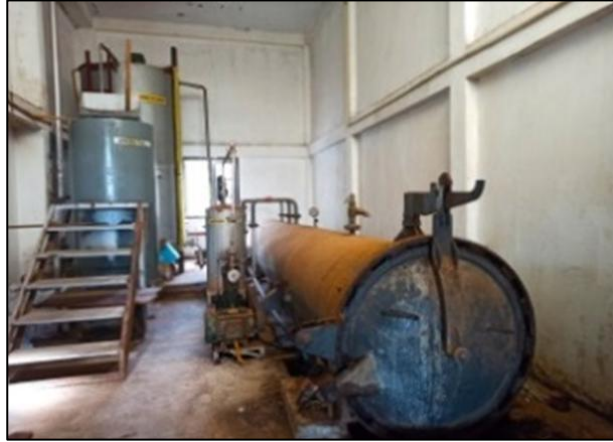
Figure 1: Impregnation plant –STC Boossa
